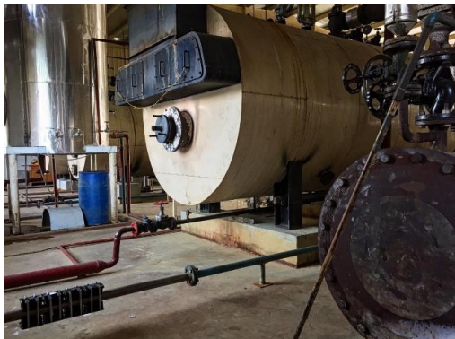
Figure 1: Boiler in the washing & dyeing plant
