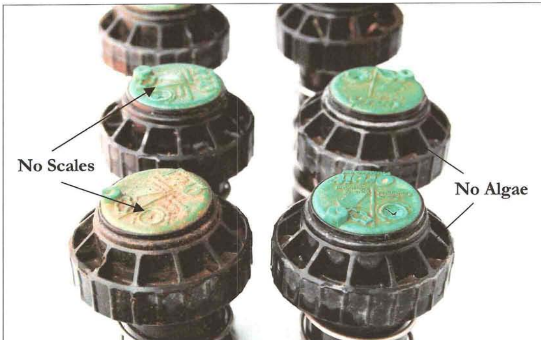
CONDITION OF SPRINKLERS AFTER 60 DAYS OF INSTALLATION (WITH GMX)
